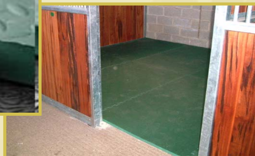
Complete Supersoft washbox installation
